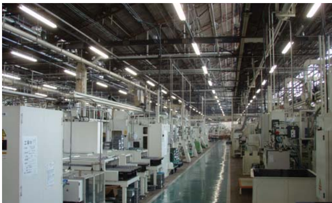
Efficient plant lighting: More efficient lighting installed
